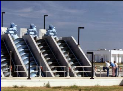
Archimedes screws pump wastewater in a treatment plant in Memphis, Tennessee, USA. Each of these screws is 96 inches (2.44 m) in diameter and can lift 19,900 gallons per minute
