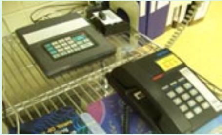
Alarming with an autodialer. Requires a phone line.
